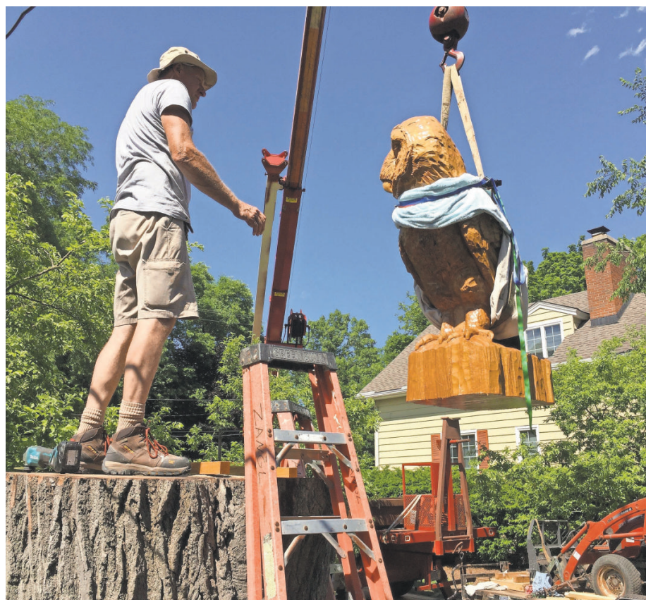
Chris Zangl of Milwaukee Landscape and Design assists in the installation of a wooden sculpture at 8125 Milwaukee Ave., Wauwatosa. The sculpture sits atop a stump left after a storm necessitated taking down a landmark tree.
